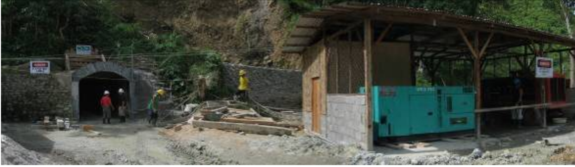
Above is the new Mafoko Portal (left) being constructed to enable mechanized operations and the powerhouse at the T'Boli gold-silver project.
