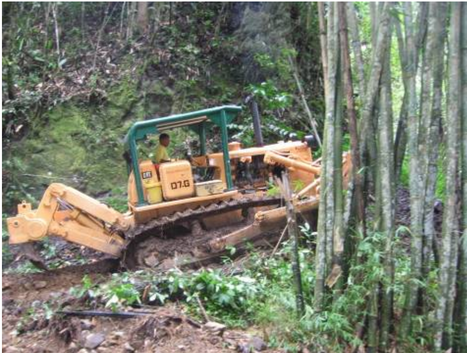
Company Bulldozer in operation clearing old tracks to improve “farm-to-market” access for the local people and for drill pads.
